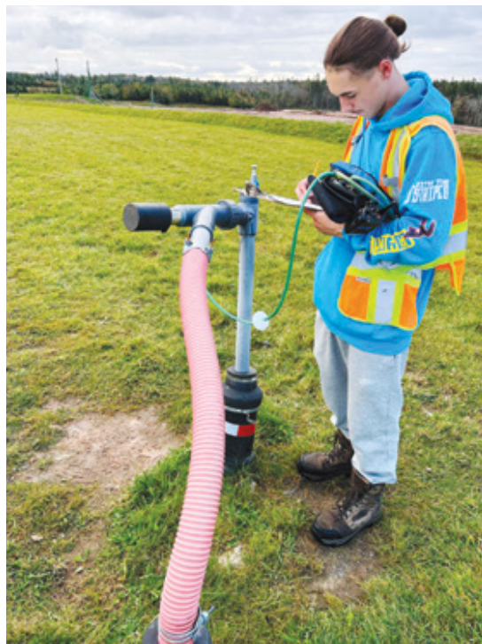
One of the six-member Gas Control System Team takes readings from a hand-held gas detector. Monitoring is round-the-clock at the Otter Lake landfill. At least one member of the team is always on duty. The device, a GEM5000™ , samples and analyzes the methane, carbon dioxide and oxygen content of landfill gas. Readings guide adjustments to the suction rates of the gas vacuums attached to each of the 75 active wellheads. Odour-causing gases formed with sulphur compounds are siphoned off and burned using the odourless and highly flammable methane gas also generated in the landfill. Photo: Jason Timms
