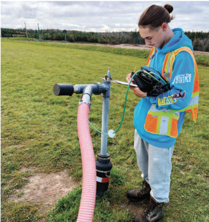
A Gas Control System Team member at the Otter Lake Landfill takes readings from a hand-held gas detector. They are used to guide the suction rates of the gas vacuums attached to each of the landfill's 75 active wellheads. Photo: Jason Timms
