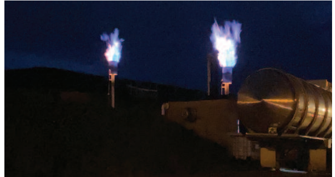
The methane gas suctioned from the garbage burial cells at the Otter Lake Landfill is being flared. The process consumes the sulfur compounds, the source of the noxious odour in landfill gas. In daylight, flares are hardly visible because of methane's nearly transparent blue flame. Photo: Jason Timms
