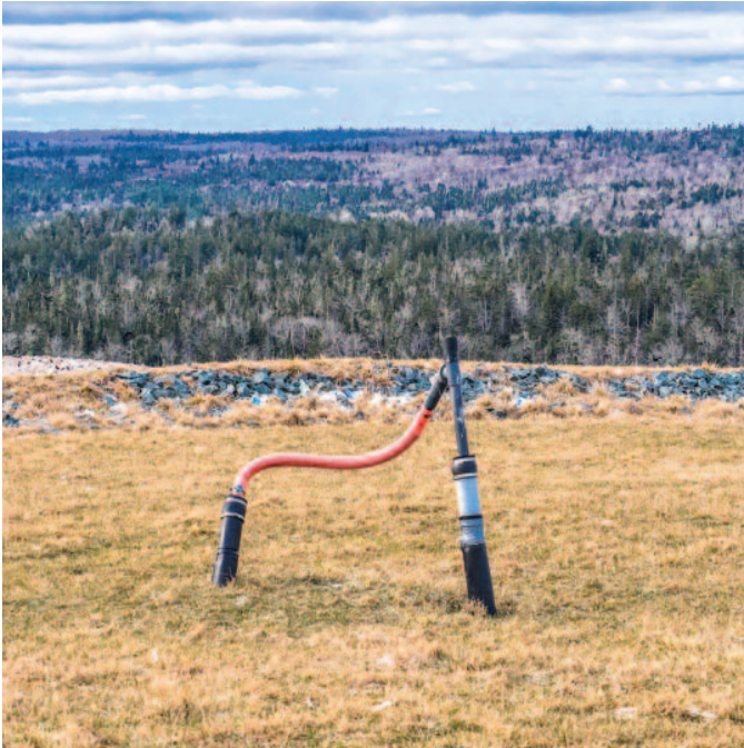
Landfill Gas extraction well
