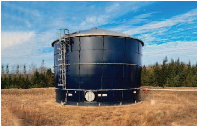
Leachate storage tank
