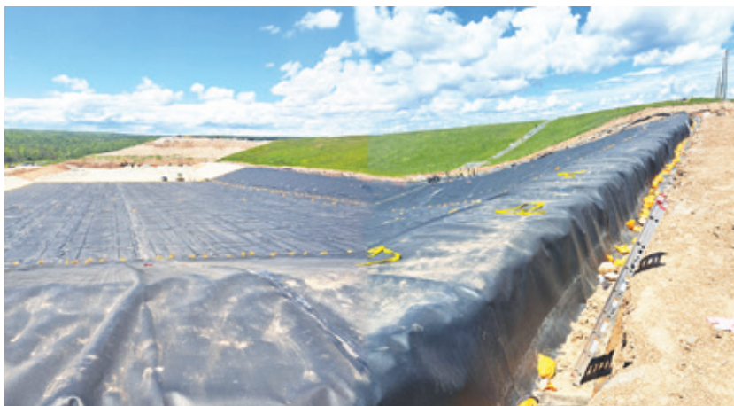
View from the top of 7B, the new cell. The base liner is shown in place, sloping to the surface where it is keyed into the ground. Photo: Scott Morash
