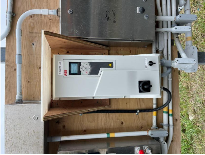
VFD at Blower 2
